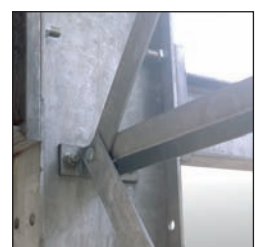
Detail of bracing connection on galvanised rack
